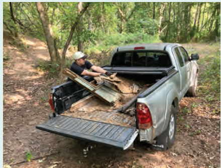
A volunteer loads leftover pieces of the old cabin into the Legacy truck for disposal.
