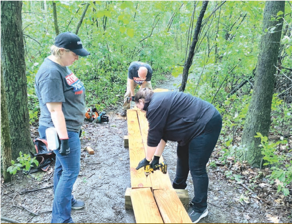
Volunteers from Scio Twp Meijer (store #173) install raised boardwalk at Lloyd & Mabel Johnson Preserve
